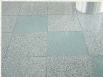
Natural stone combined with glass panel adds a special touch to every entrance hall.
